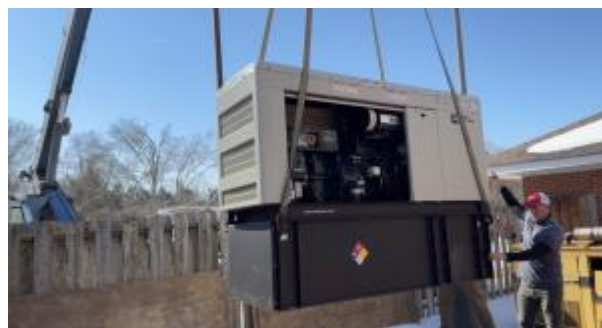
Cummins diesel generator installation at Shelby County Fire Station 61 in Eads, Tennessee
