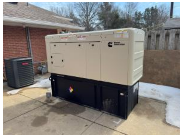
Completed installation of a Cummins diesel generator at Fire Station 61 in Eads, TN.
