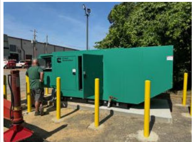
View of Cummins generator installation at UKG-Memphis
